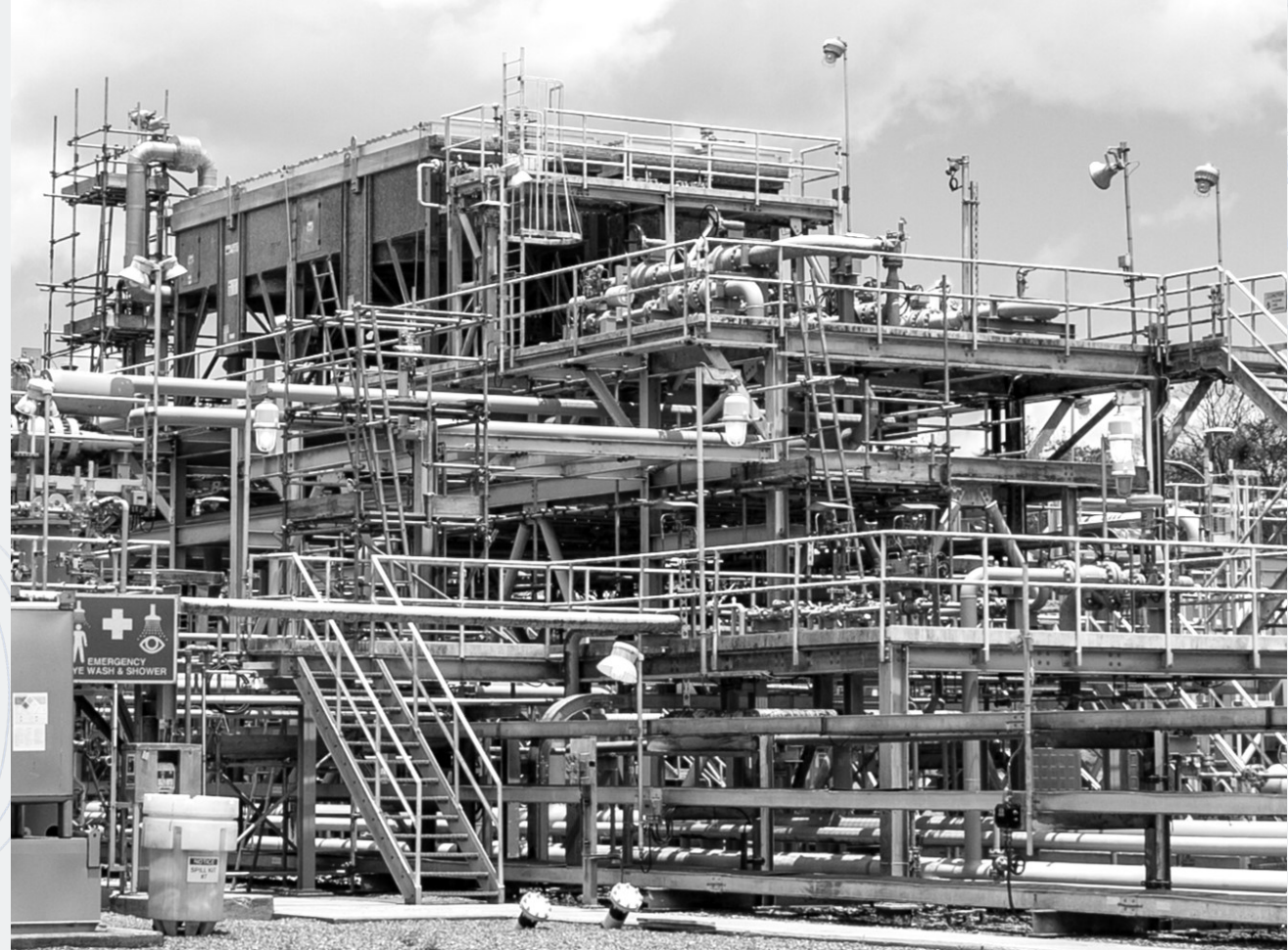
Evergreen Natural Gas Facility, Central Block
